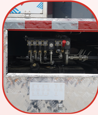
Ground Panel Operation
